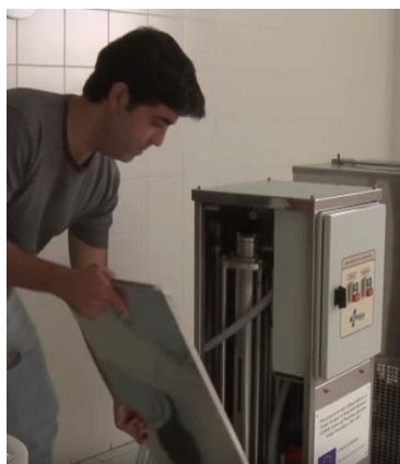
Imagen 2: Installing the disinfection device inside commercial equipment
